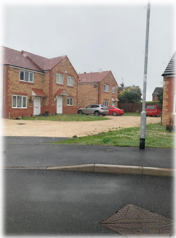
Figure 29: View of poor quality surfacing to a cul-de-sac
