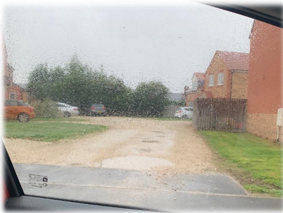
Figure 28: View of poorly surfaced access to cul-de-sac with surface water
