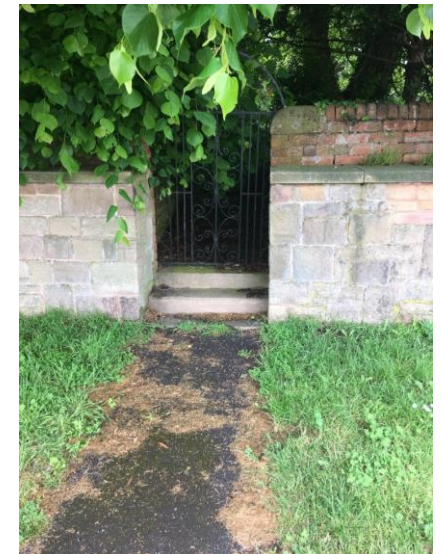
Riverlyn House. The protection in the defensive walls from flooding is lacking here in a secondary access to the property
