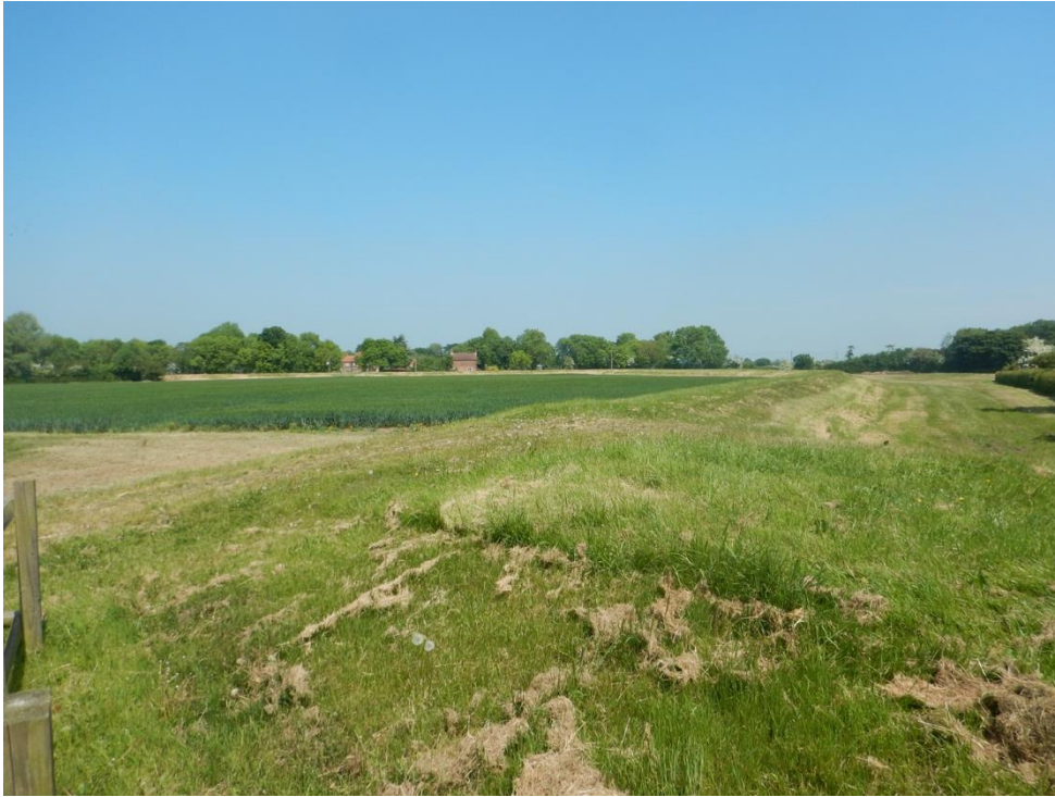
View opposite River Trent Car Park, showing the flood bank and footpath to Fiskerton Mill.
